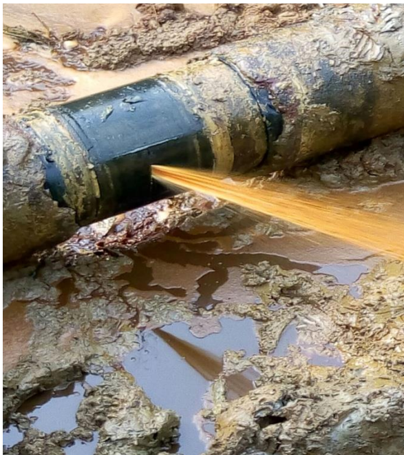
spill point before repair
